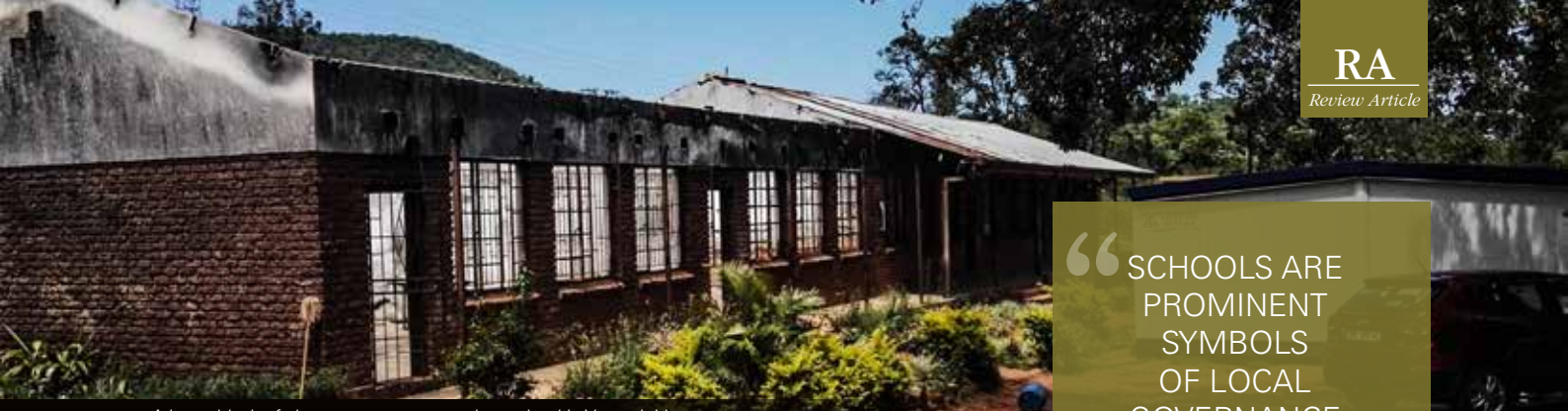
A burnt block of classrooms at a secondary school in Vuwani, Limpopo
